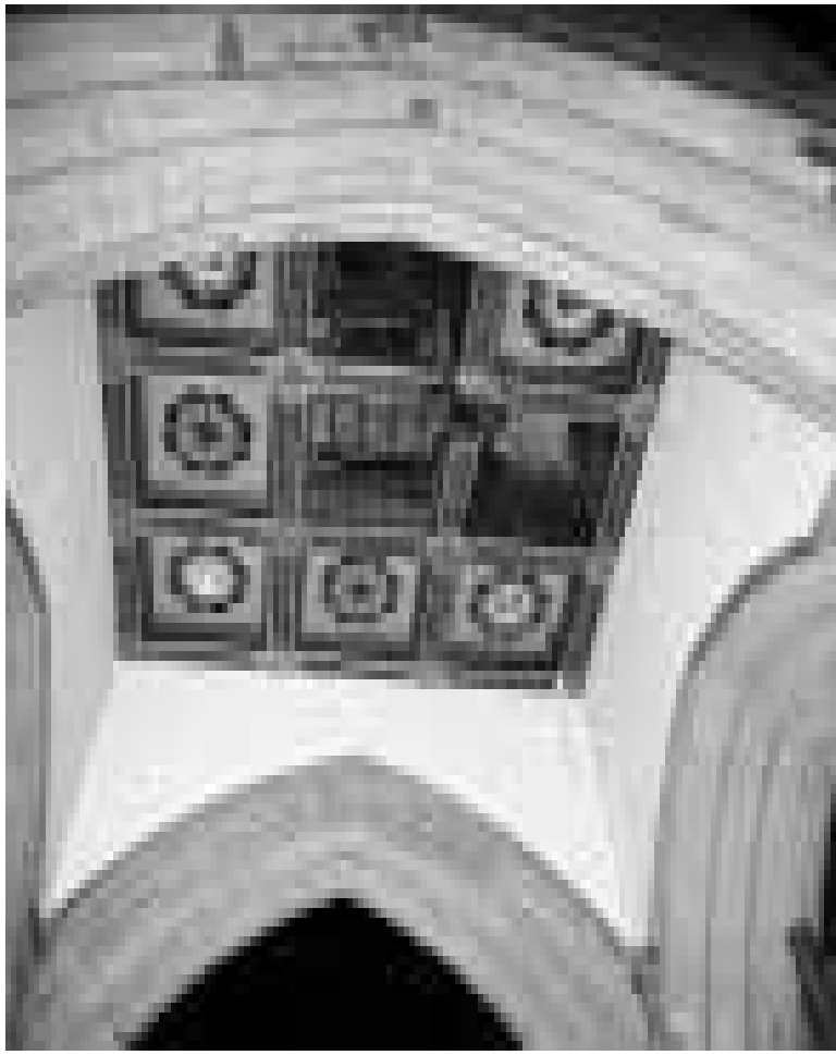
Long view of the damaged chancel ceiling.
