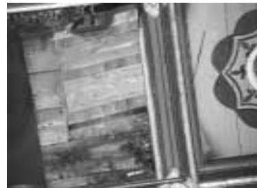
Close-up view of charred beams.
